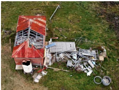
The oil store is sorely in need of repairs
